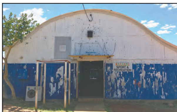
DISREPAIR: The Sport and Recreation building.
